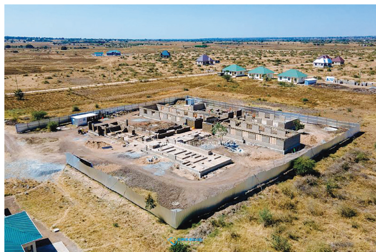
This image was captured from above during the early stages of construction of Tanzania's first standard Neonatal Care Unit, located in Kwimba District. This is another milestone of DMF commitment. Photo: Courtecy.
